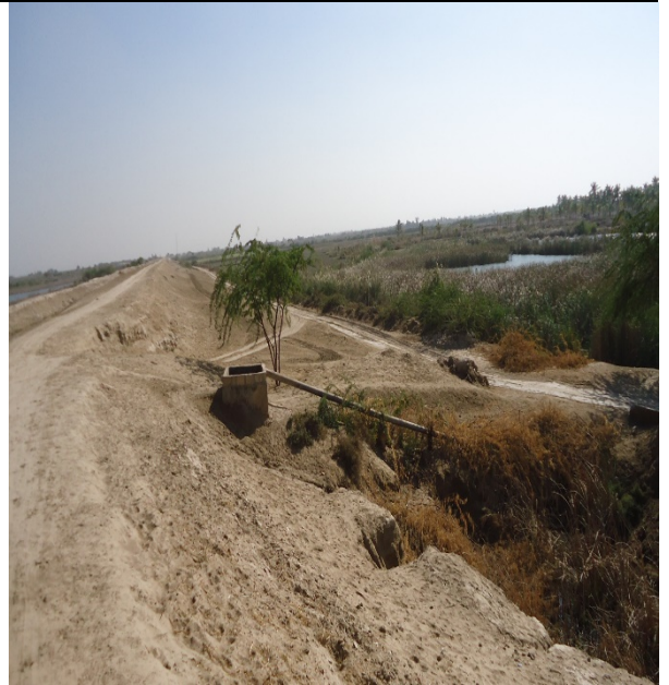
Pic 2: Land side of Bund
