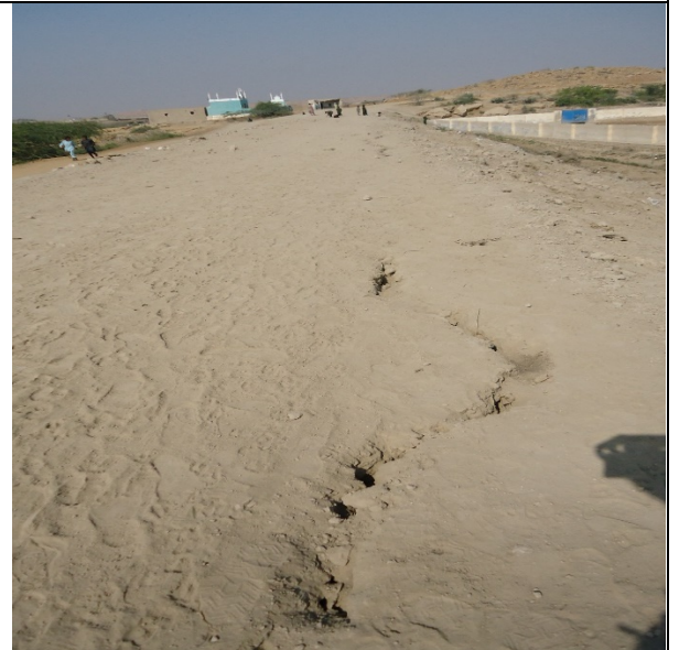
Pic 4: Damaged Area of Bund
