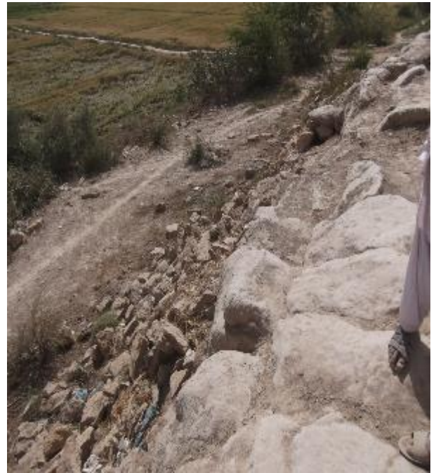
Damaged stone pitching at 151/1
