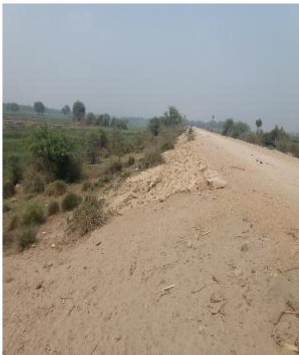
Damaged Stone pitching at 123/3 of SM Bund
