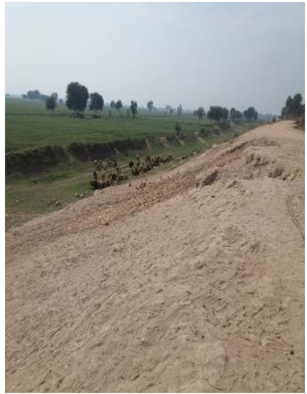
Damaged stone pitching at 127/3
