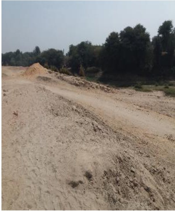
Condition of Embankment at 126/4
