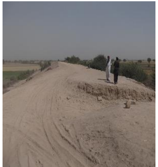
Condition of embankment at 150/2
