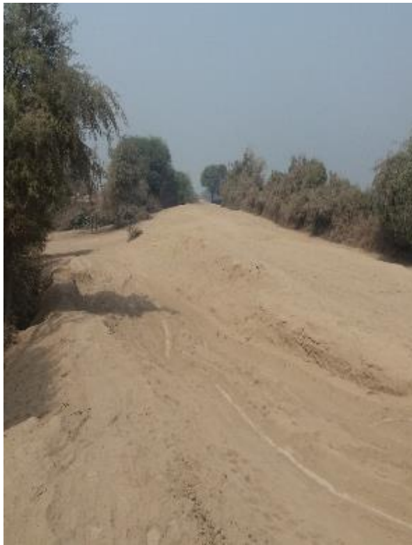
Condition of SM Bund at Mile 123/0
