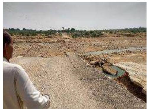
Effects of Flood at Dhari Shrief Dam site area
